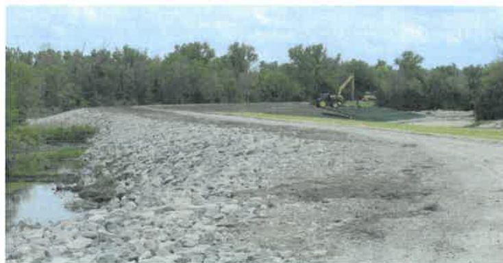
Lower Platte North NRD makes repairs on Clear Creek in May, which was breached during the 2019 flood.
