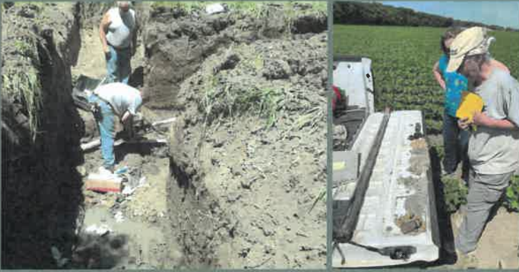
Above left: Lower Niobrara NRD makes FEMA repairs on the West Knox Rural Water System, which was damaged during the 2019 Bomb Cyclone. Above right: Sue Lackey, Conservation and Survey Division, records data from samples collected with a geoprobe in Cedar County.
