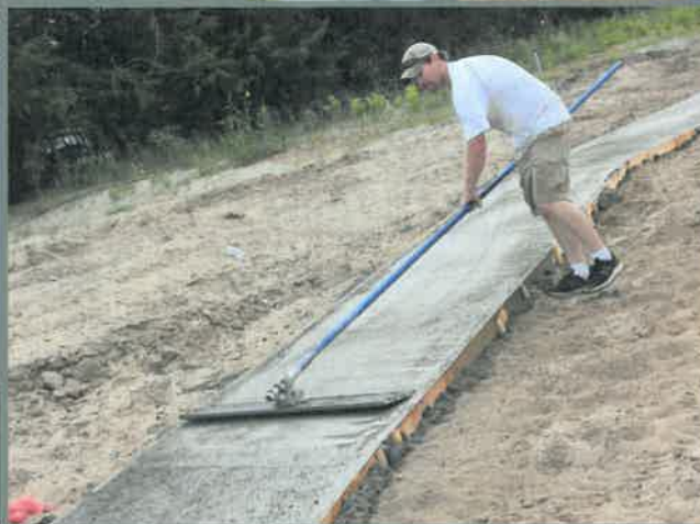
Above: Upper Loup NRD Resources Technician Shane Young smooths cement for a walking path at the new Arboretum in Theford near the District office.
