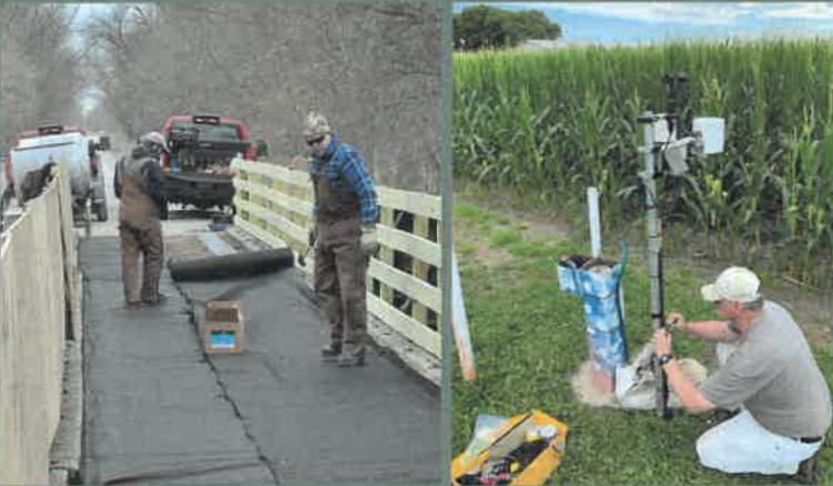
Above left: Repairs are made on Lower Platte South NRD's Homestead Trail Bridge south of Lincoln. Above right: Russell Oakland, Lower Platte North NRD lead water resources specialist, installs a solar-powered METOS weather station.
