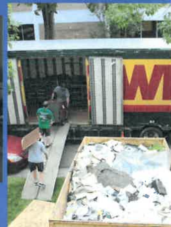
SERVPRO moves out NARD office furniture to determine if it can be cleaned and salvaged.
