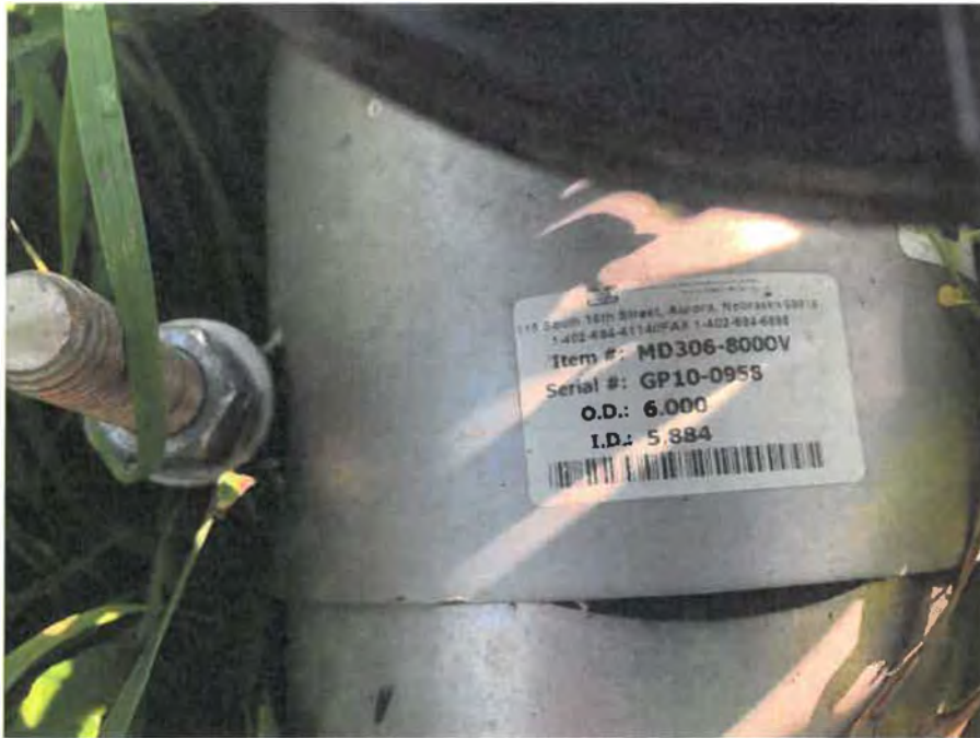
Figure 1: Photo of Meter Serial # on Well Reg: G-042047 (September 19, 2022)
