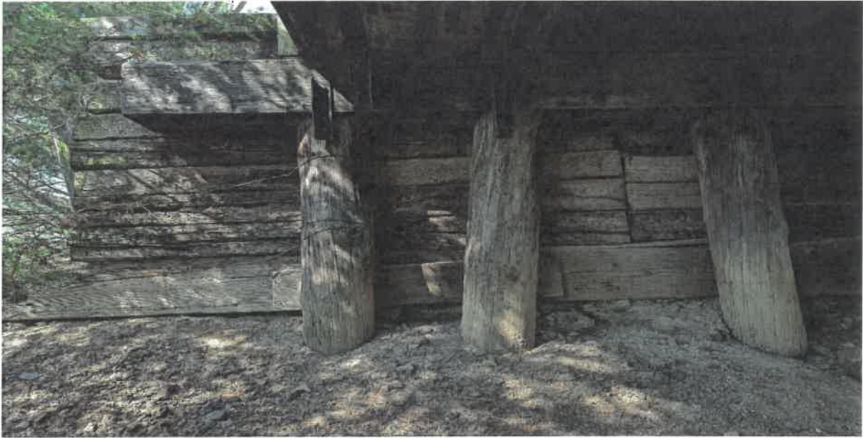
Backwall plank separating and deteriorating
