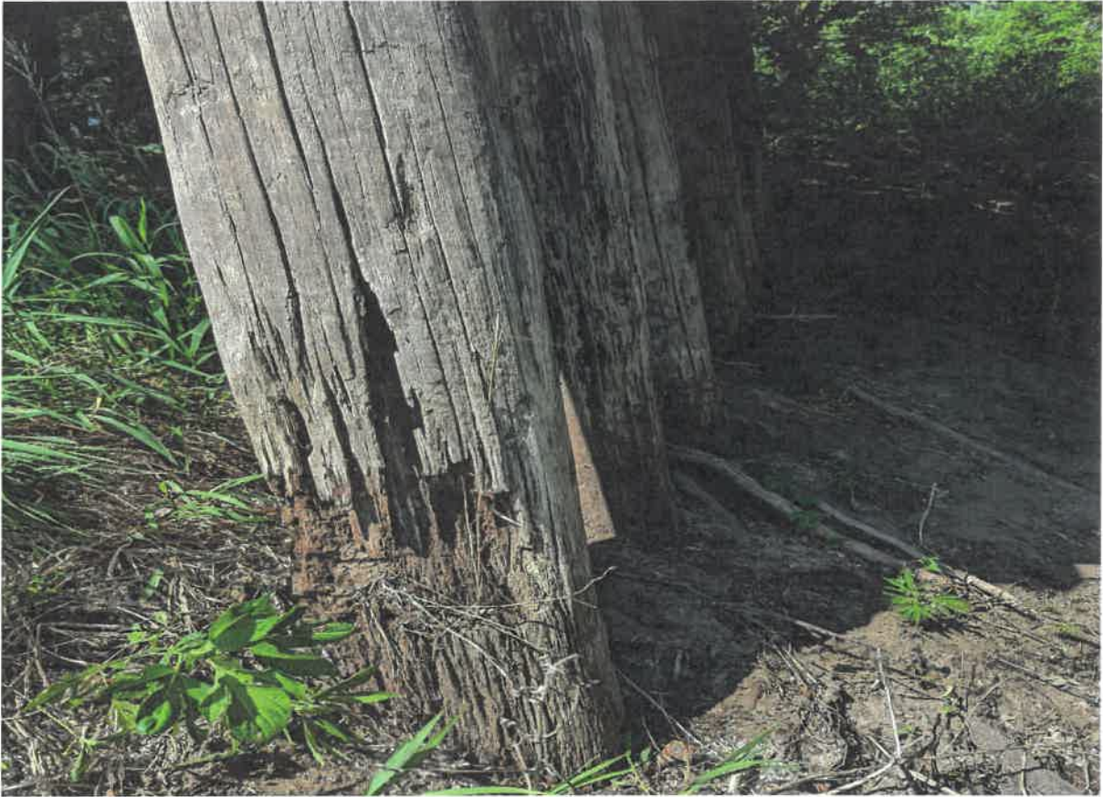
Example of damaged pile that needs to be replaced, Bent 4
