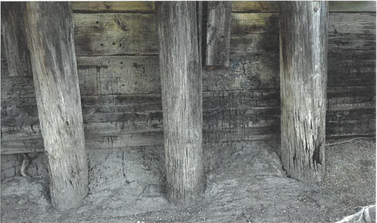
Ruined pile and undermined backwall
