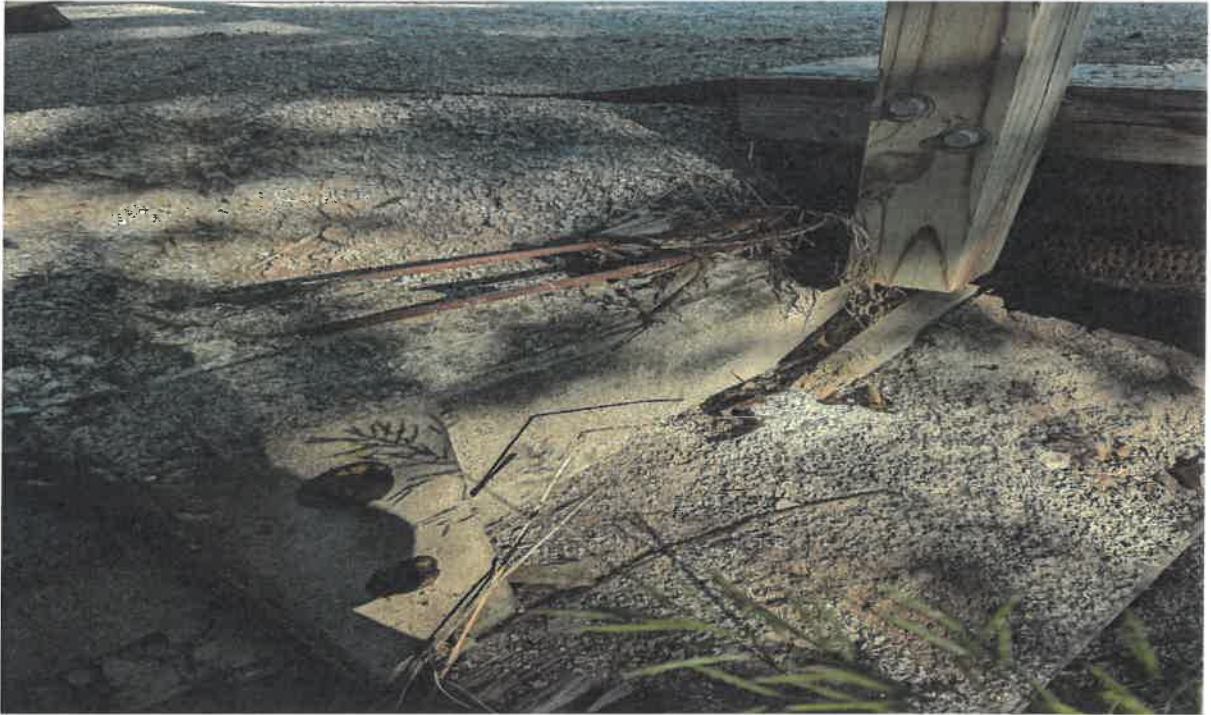
Broken concrete backwall
