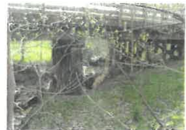
Figure 7-17: Trail Bridge with exposed footings.
