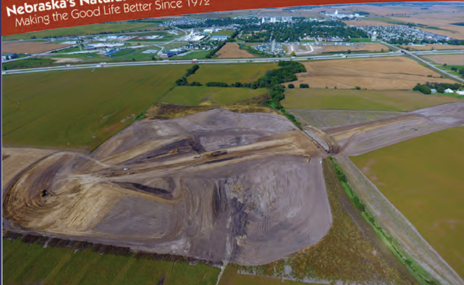
This dry dam along Ash Hollow Creek, south of Waverly, will be completed in the spring. The NRD and the City of Waverly are each funding half of the nearly $3 million project cost. It will control flooding in the town and remove about 90 properties from the floodplain. Flood insurance would no longer be necessary in order to get loans to buy those properties. The dry dam will only hold water after a storm, releasing it at a controlled rate.
