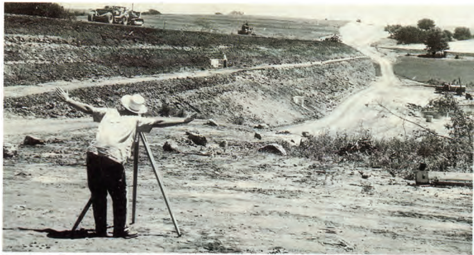
Project Engineer Lew Kehne directs construction of an Upper Salt Creek flood control structure in 1954.
