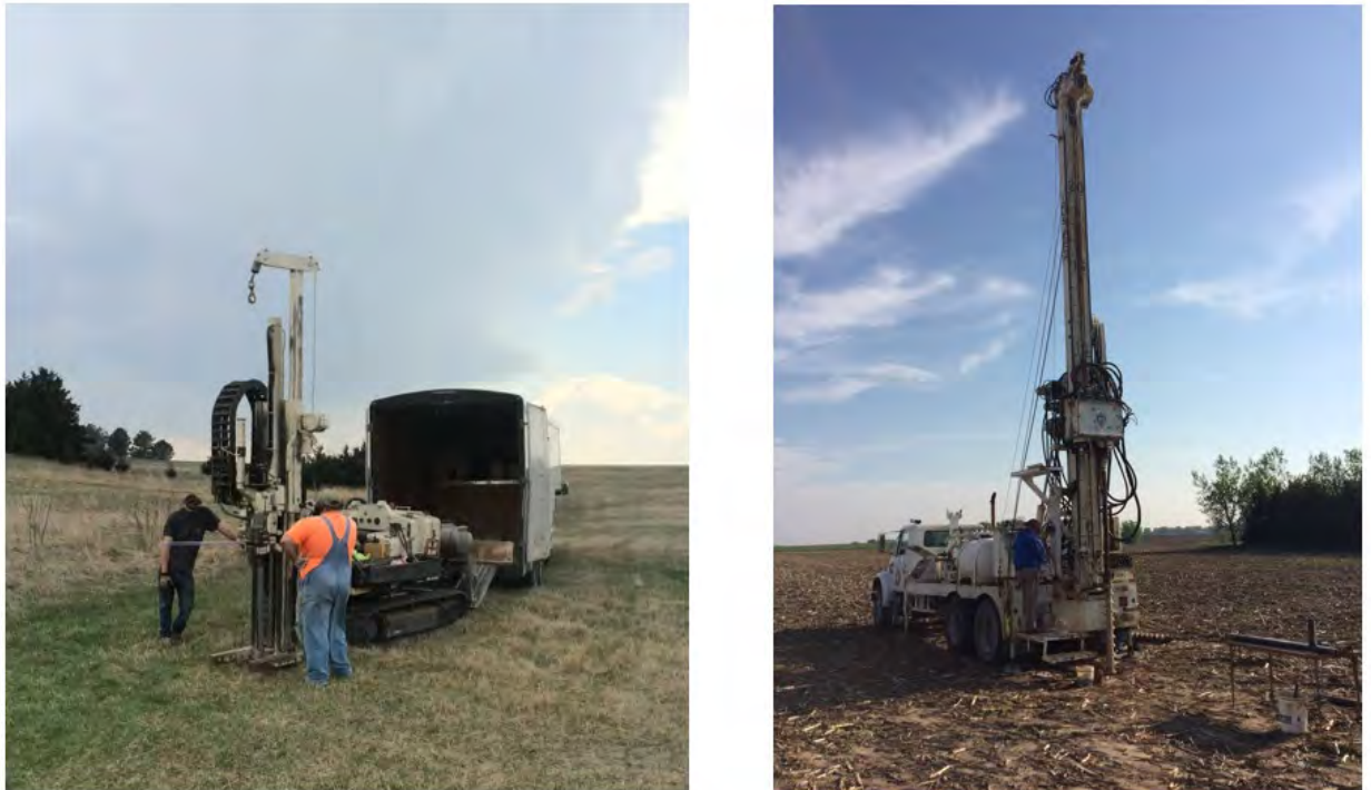
Figure 14 – Geoprobe® (left) and Rotary Drill Rig (right) Used in Vadose Zone Sampling
